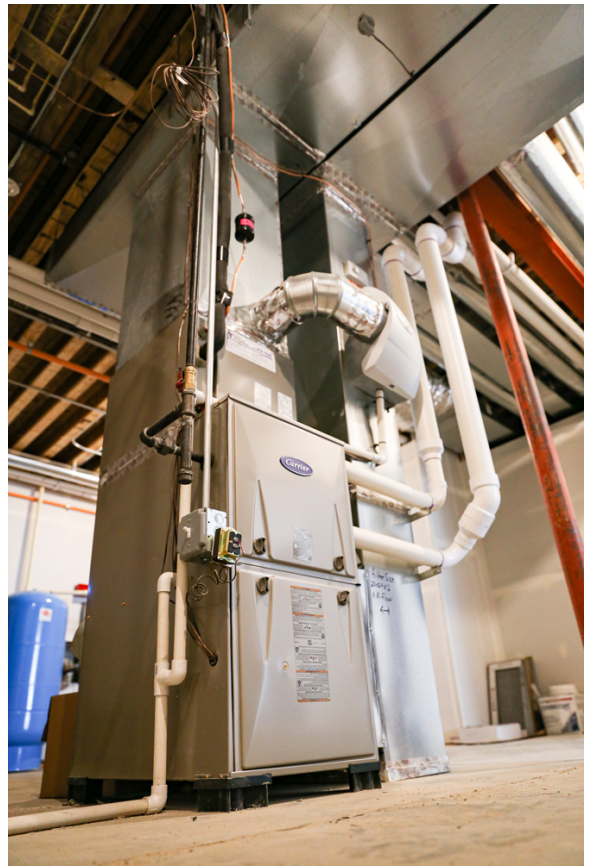
Behind the scenes: a look at the mechanical room during construction in the Elm Estates home by Icon Building Group, featuring Carrier HVAC equipment
